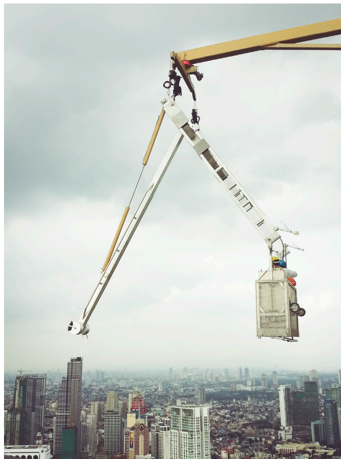
Machine with pantograph in the cradle to reach internal areas of the facade. Installed in Makati's yellow tower, in Makati, Philippines.
