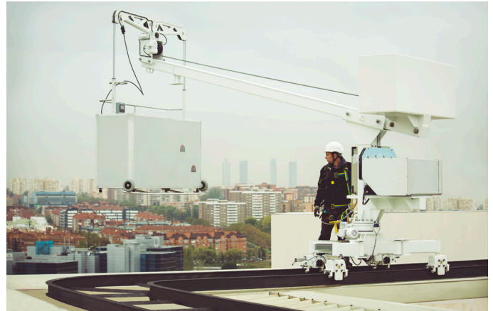
FBA 1 B.M.U. installed in Spain. The machine design is optimized making it lightweight and inconspicuous in the building roof, in a custom color as per client's requirements.
