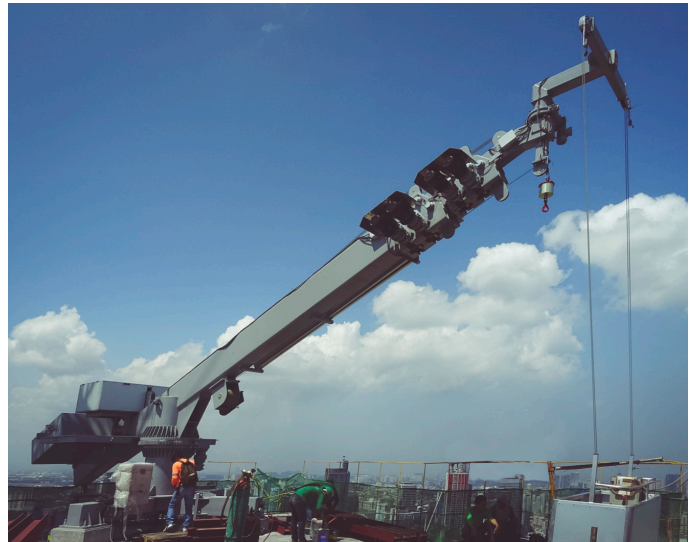
Trump Tower: a compact FBA S machine stationary and through slewing all facades can be reached confortably. Installed in Manila, Philippines.
