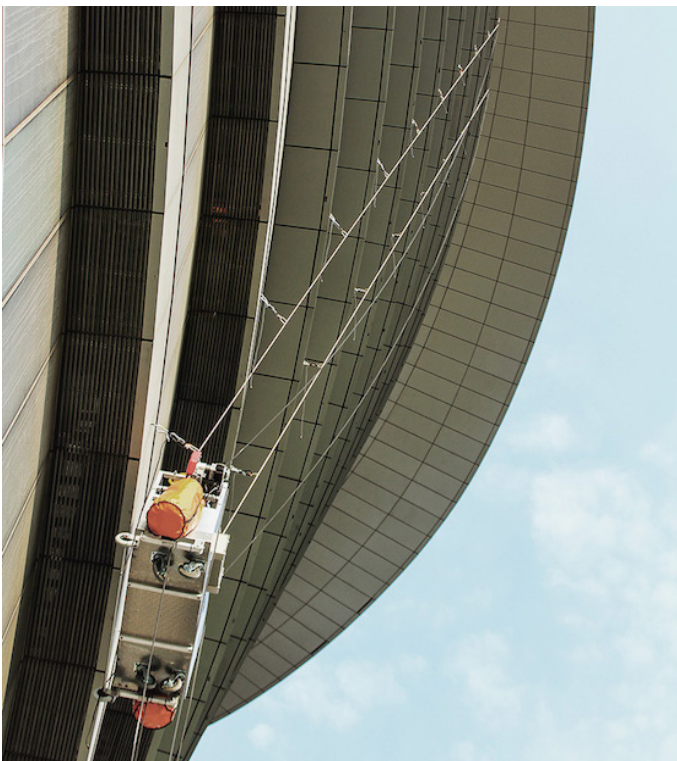
Facade restraint pins to keep the cradle next to the facade.
